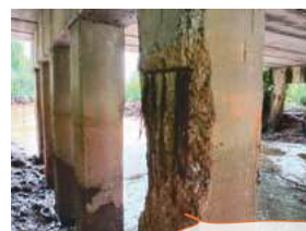
Bridge pier deterioration due to salt exposure
